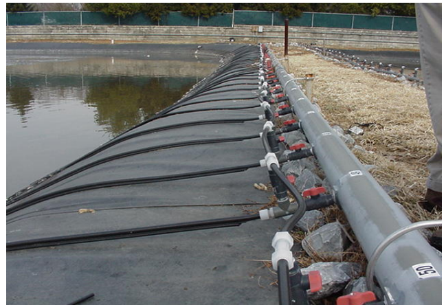
High efficiency diffused aeration
