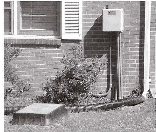
HYDRAULIC UNIT AND CONTROL INSTALLATION
